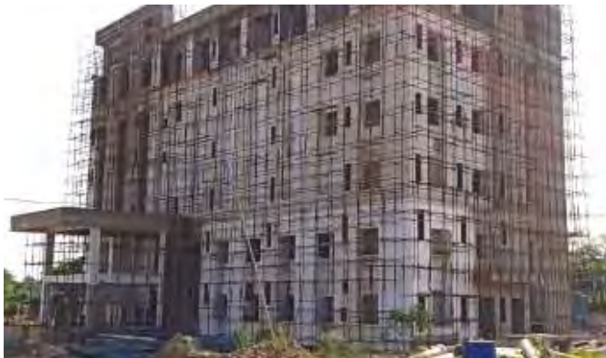
ROURKELA SMART CITY PROJECT ODISHA- COMMAND CONTROL CENTER
