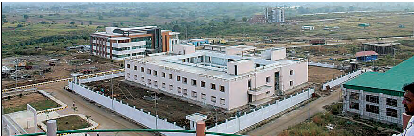
Construction of Permanent Non Residential Building for ITBP, Jabalpur, M.P. -Aerial View
