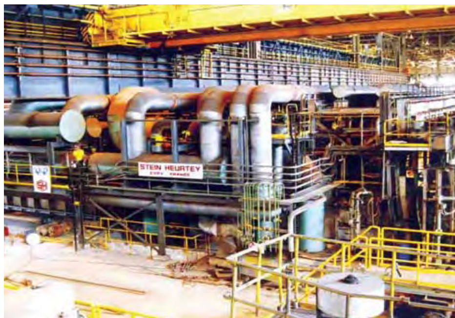
Walking Beam Furnace at Vizag Steel Plant, Vizag
