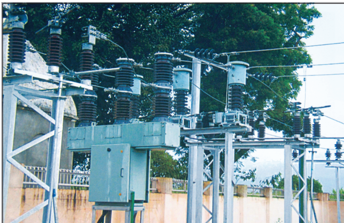
33kv Sub Station in Uttar Pradesh
